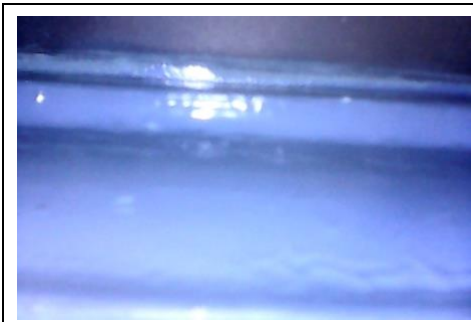
The first view seen with the fibre-optic cable camera – the glazing bars of the original partition.
