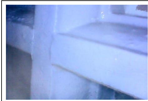
Both the vertical and horizontal glazing bars can be seen in this view, along with the glass still intact.
